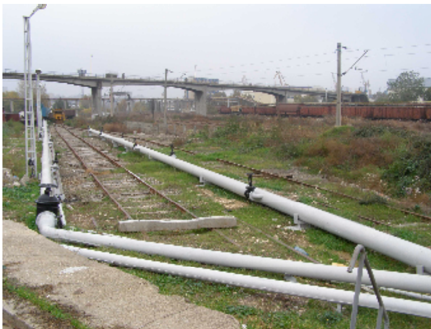
Foto: Conducte transport biodiesel
